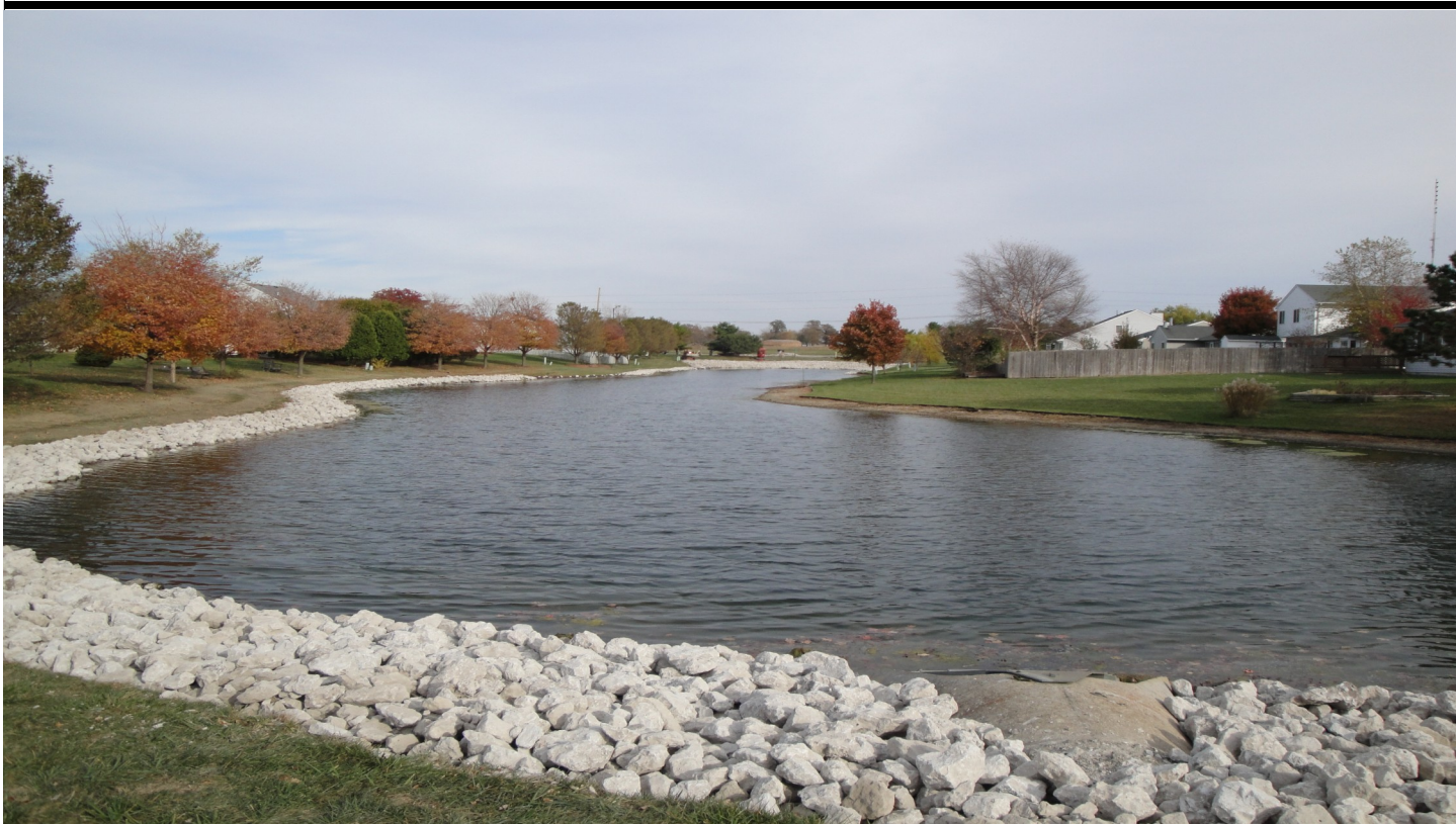
View of long basin from Alpine Drive looking East (work in progress)
